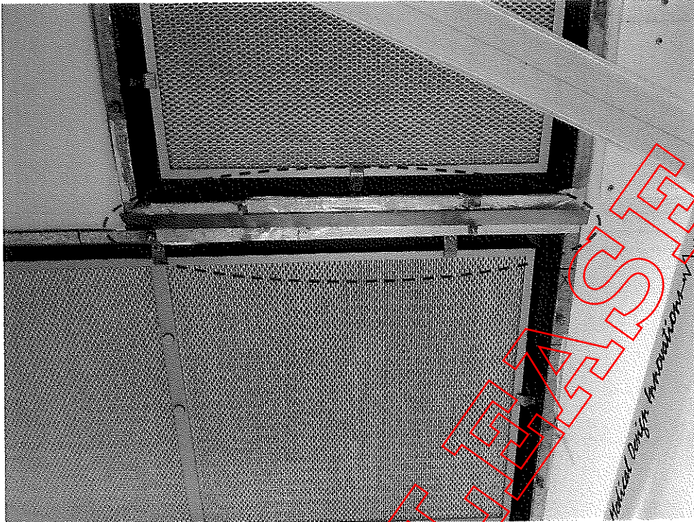
Photo 1: Example of the use of foil tape and inadequately secured strips of stainless steel to fill the gaps between the HEPA filter modules.
